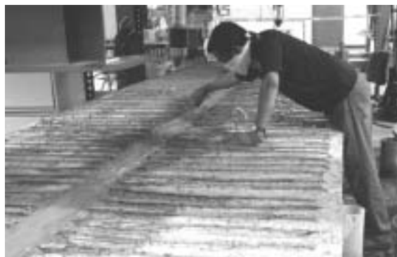
Fig. 10—Filling of gap between Box Beams BBD-I-1 and BBD-I-2 of Bridge Model BBD-I with structural concrete.
