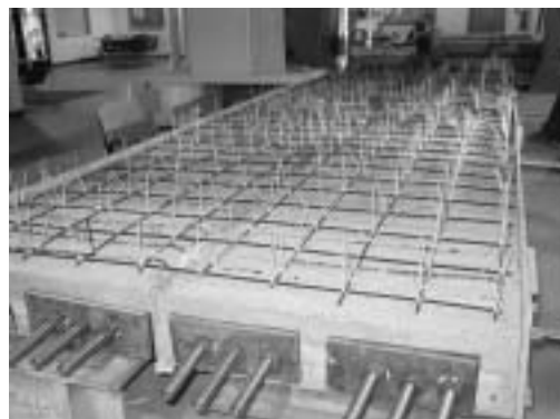
Fig. 11—CFCC reinforcement cage placed in deck slab formwork of Bridge Model BBC-I.
