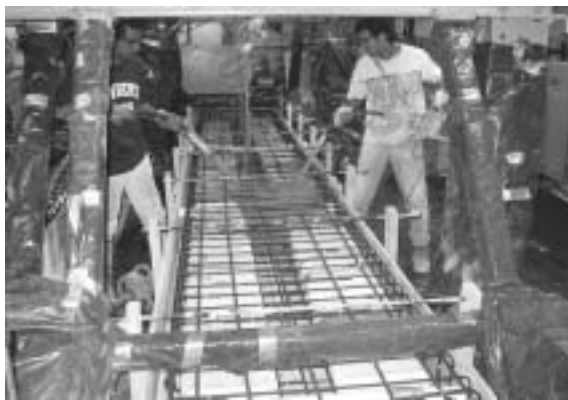
Fig. 8—Placing of concrete and use of vibrating equipment for proper compaction of concrete in Box Beams BBC-I-1 and BBC-I-2 of Bridge Model BBC-I.
