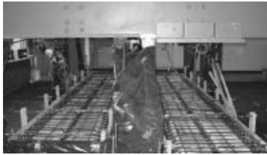
Fig. 5—CFCC reinforcement cage placed in formwork along with pretensioning strands for casting two box-beams for Bridge Model BBC-I.
