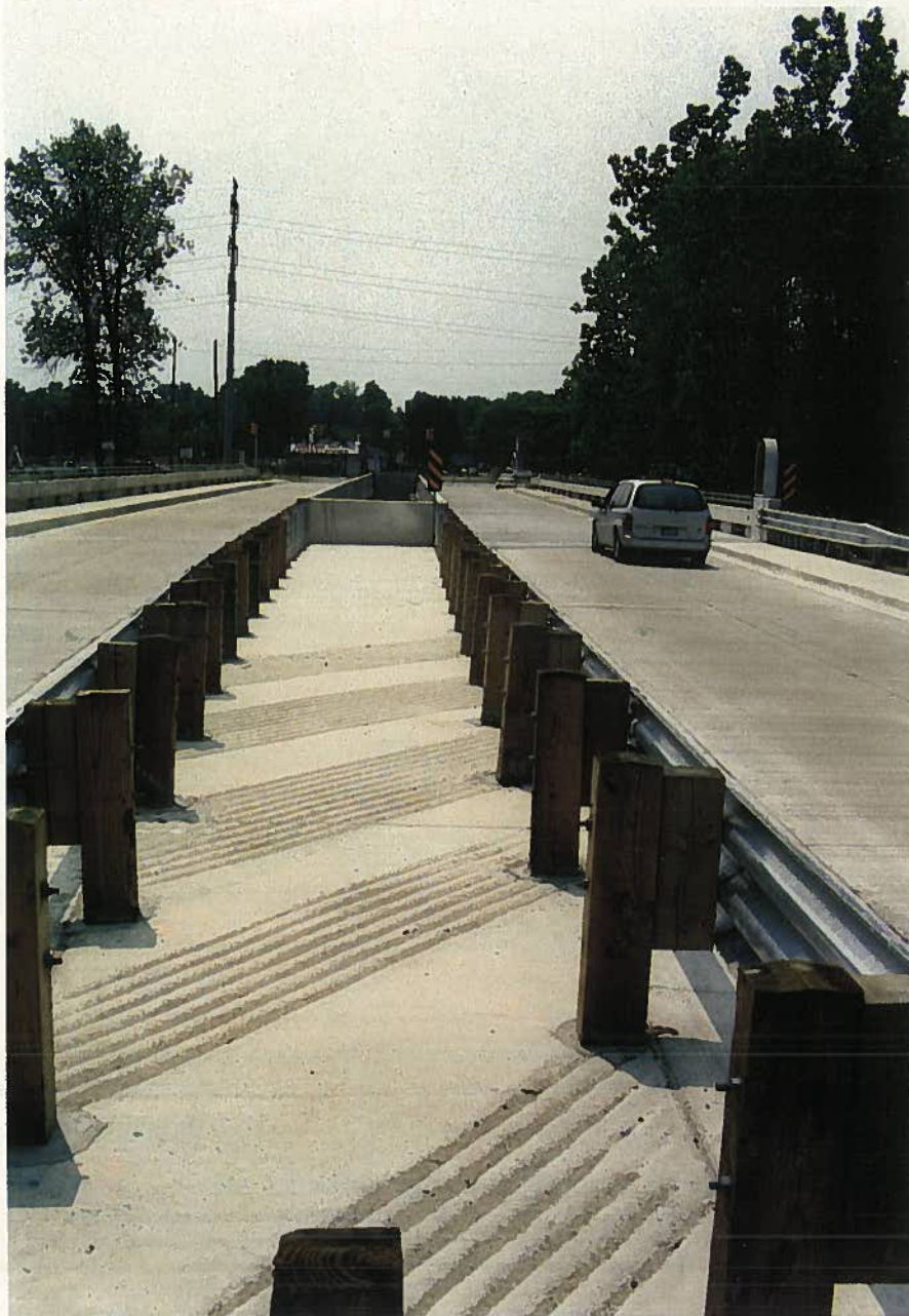
Fig. 1a. Southward view of Bridge Street Bridge, Southfield, Michigan. CFRP structure, Structure B, is on the right.
