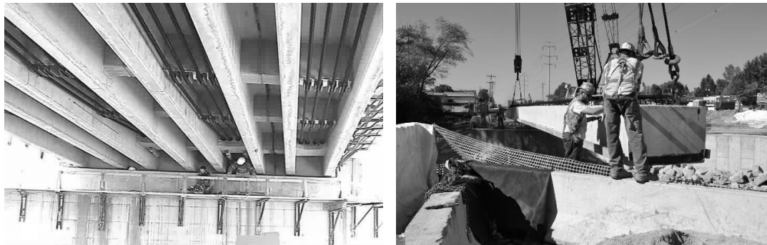
Figure 1: Left: Bottom view of Bridge Street Bridge. Right: Construction of M-102 Bridge.
