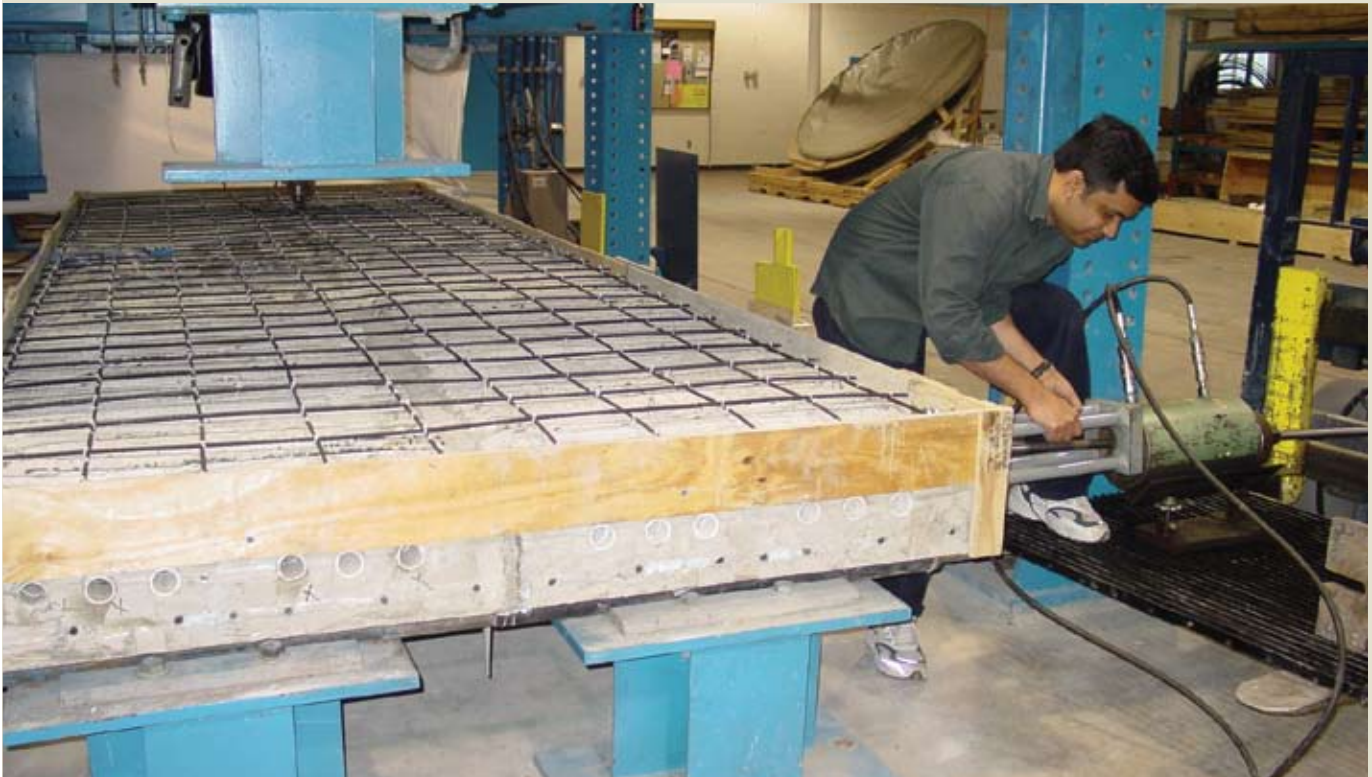
Figure 16. This carbon-fiber-composite cable reinforcement cage made from square grids of 0.3-in.-diameter (7.5 mm) strands at a constant spacing of 8 in. (200 mm) was the deck-slab reinforcement.
