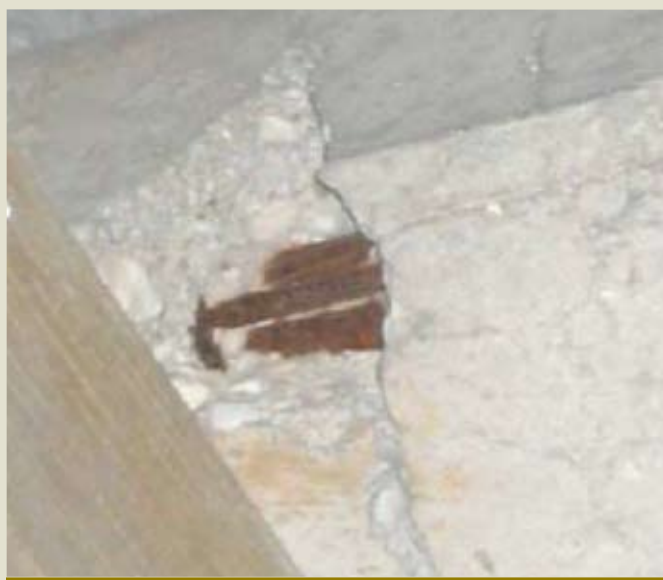
Figure 2. This steel-reinforcement corrosion resulted after its concrete cover experienced spalling.
