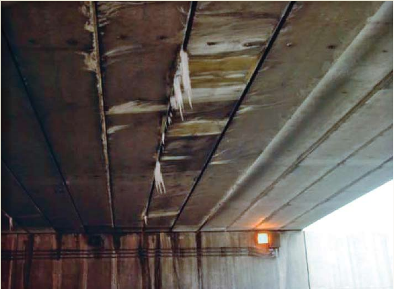
Figure 3. Water that has formed icicles can easily infiltrate longitudinal cracks that develop between adjacent box beams.
