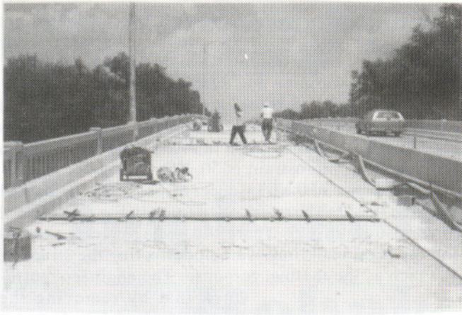
Fig. 4 — Asphalt deck replaced by white silica-fume concrete. Note the bridge is still open to traffic.
