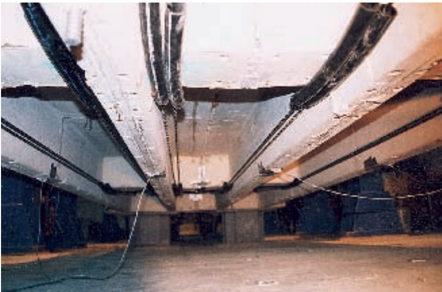
Fig. 3. Post-tensioned continuous externally draped CFRP Leadline tendons (shown from below), Bridge Model CDT1.
