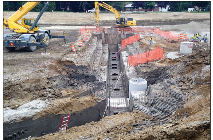
During the 167-day reconstruction project, MDOT constructed this 48-inch prestressed concrete water main under I-96, just west of Middlebelt Road in Livonia, for anticipated future use.
