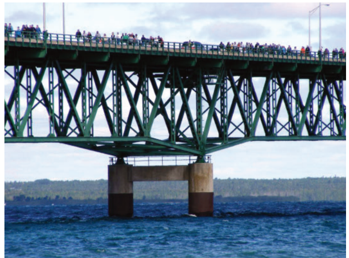
This photo of the Mackinac Bridge by Lawrence Tech graduate student Delia Radbata captures the beauty of the open web trusses that help maintain the stability of the deck despite the strong wind patterns in the area.
